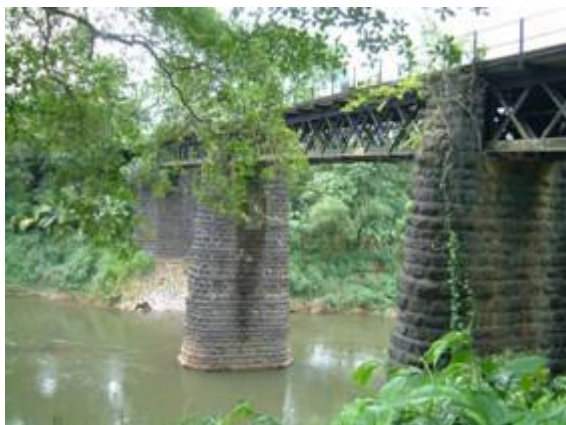
SITAWAKA BRIDGE There are many remains to be seen along the course of the dismantled narrow gauge lines. This bridge at Sitawaka used to carry the Yatiyantota branch over the Kelani River and is now used by a local road. [DH, 2 May 2004]
