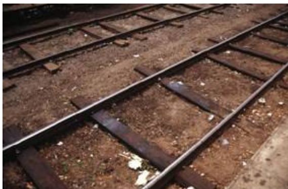
NEWLY LAID SLEEPERS AT VALAICHCHENAI (2002) With the coming of peace talks and the implementation of a cease-fire, the Batticaloa Line was reopened from Polonnaruwa to Valaichchenai. However, shortage of material meant that the sleepers were spaced with large separation from Welikande to Valaichchenai and the rail only secured directly to the sleepers by bolts without the use of clips, etc. Since this photograph was taken the BCO line has been re-opened right through to Batticaloa. [DH, 26 Jul 2002]
